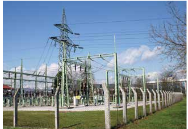
Perimeter protection ✕ Laser scan / Outdoor PIR detectors
